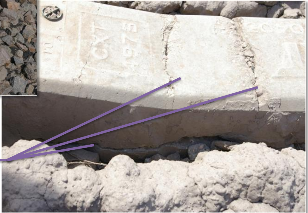
Cracked Tie (moment cracks)
