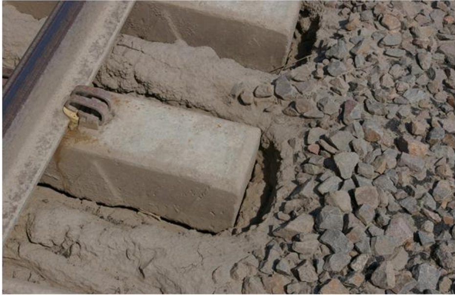
Muddy Ballast, tie cavity Indicative of tie movement/slack
