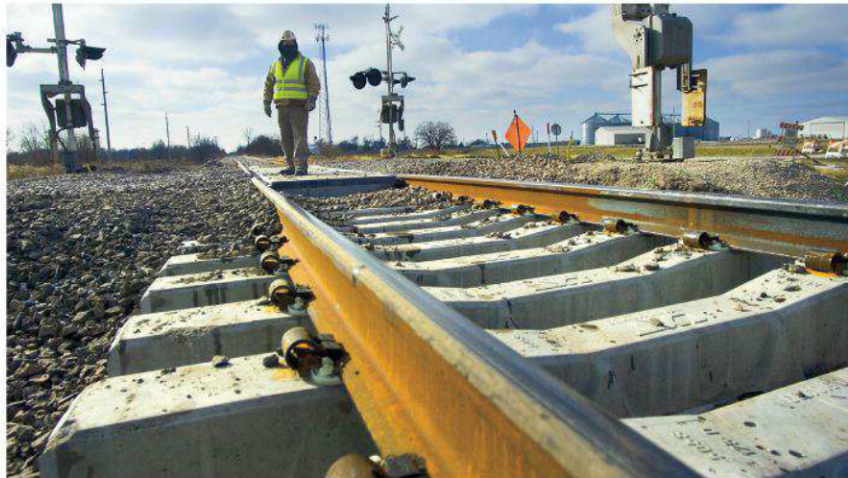
A Union Pacific worker stands guard at a grade crossing with newly laid and installed concrete ties between Williamsville and Elkhart, Ill., in December 2010. Steve Smedley
