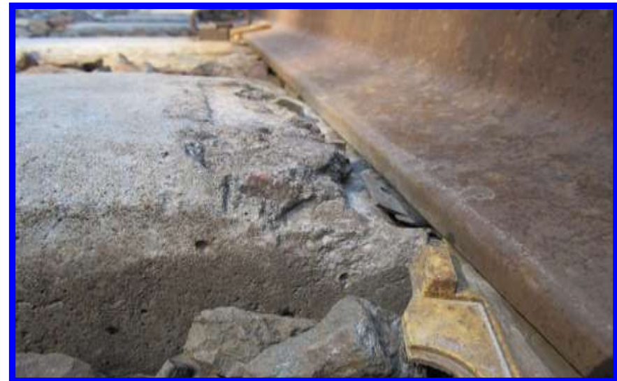
Profile view of damaged rail seat
