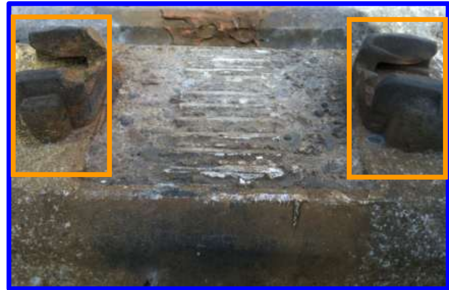
Plan view of deteriorated rail seat
