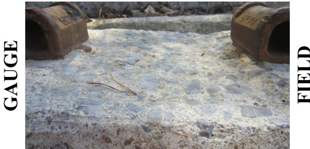
FIGURE 1 Typical wear pattern of rail seat deterioration (RSD).
