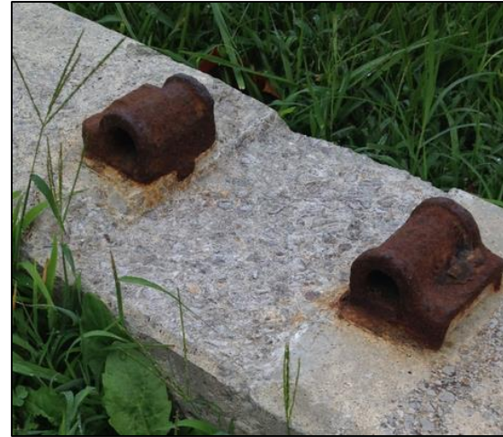
Rail Seat Deterioration
